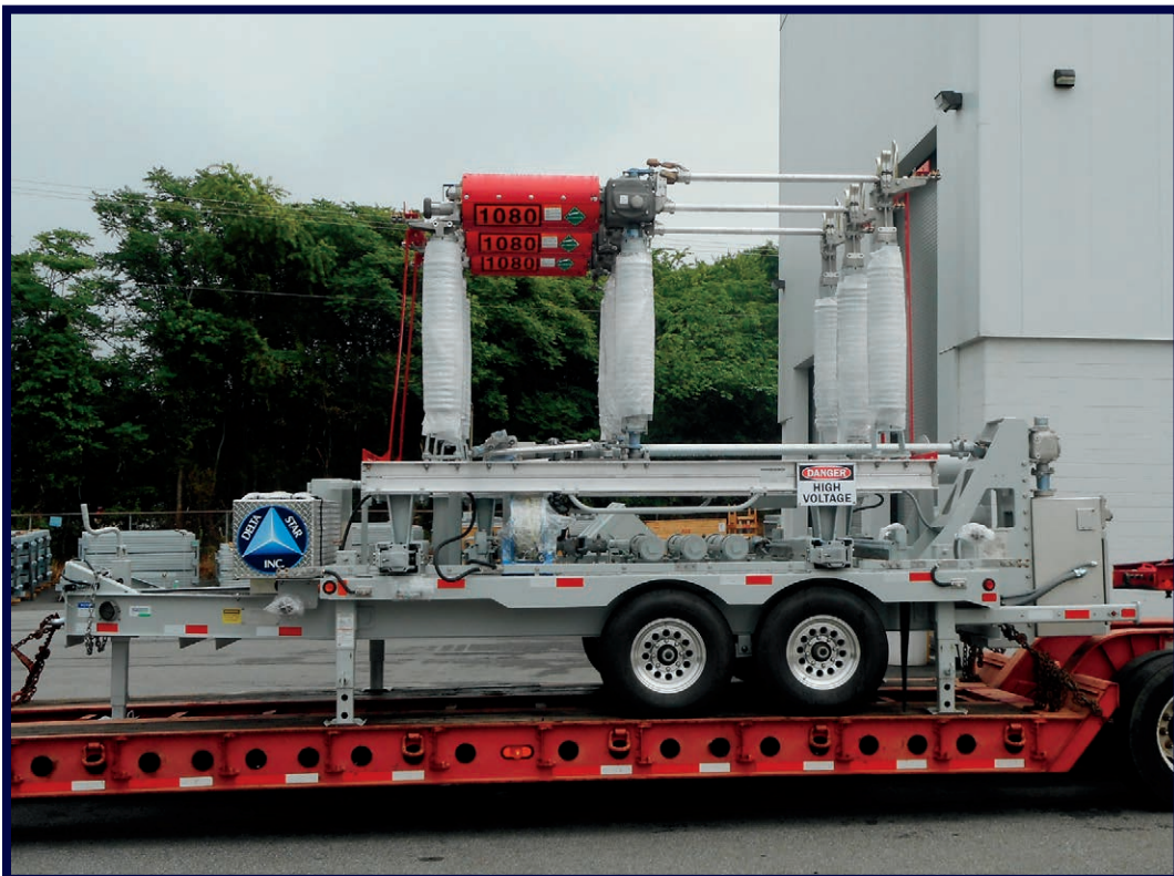
Mobile Circuit Switcher Trailer Customer Region: SOUTHEAST
