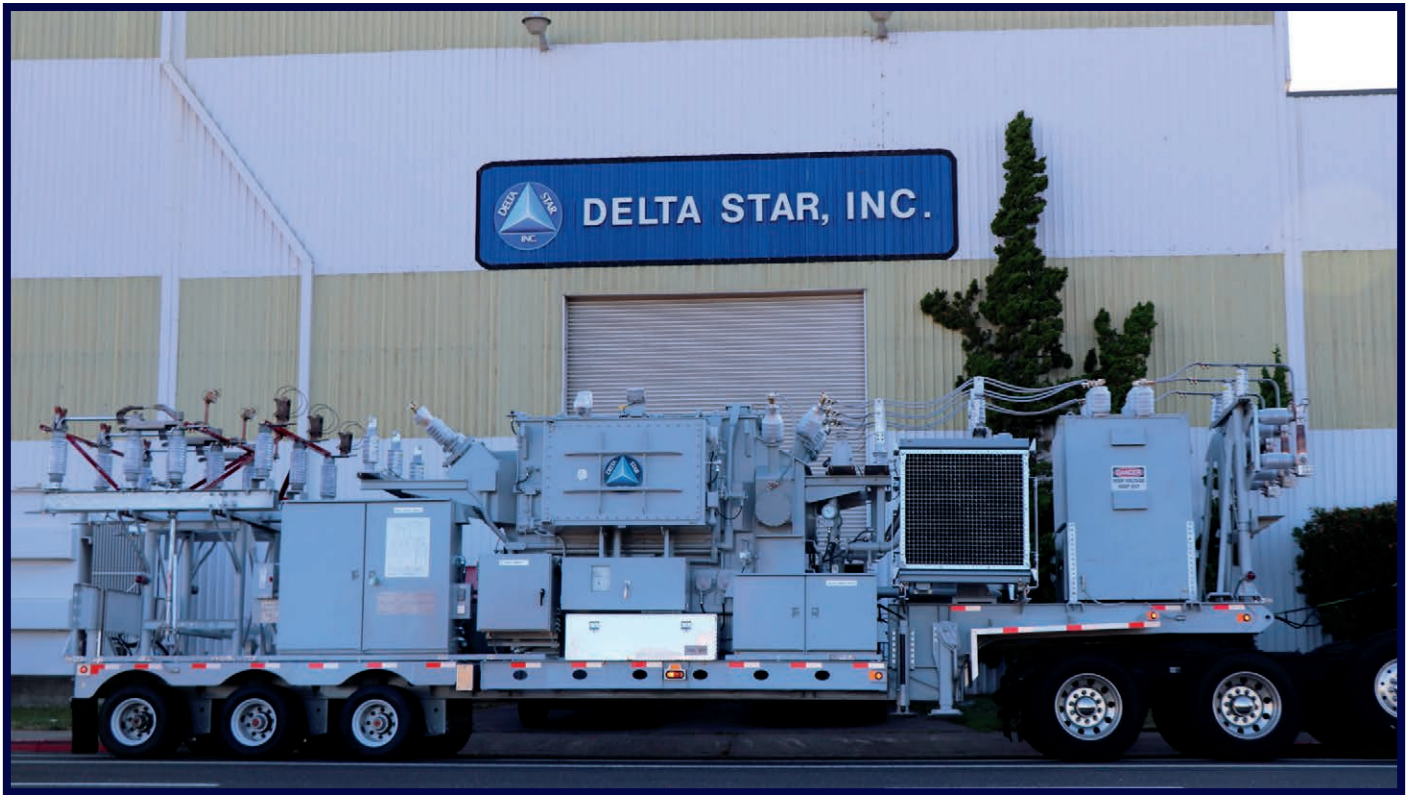
(20 MVA, 34.5 kV - 13.2 kV, LTC) 2019 | 40' | 98,000 lbs. Customer Region: WEST
