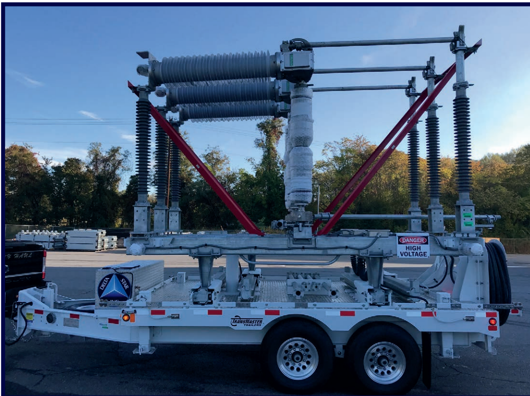
Mobile Circuit Switcher Trailer Customer Region: SOUTHWEST
