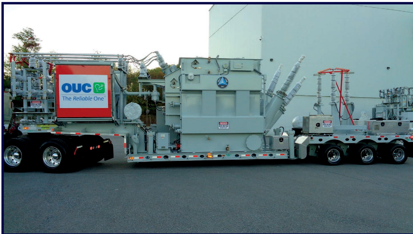
(30 MVA, 115 kV - 24.94 kV, LTC) 2017 | 46' | 127,000 lbs. Customer Region: SOUTHEAST
