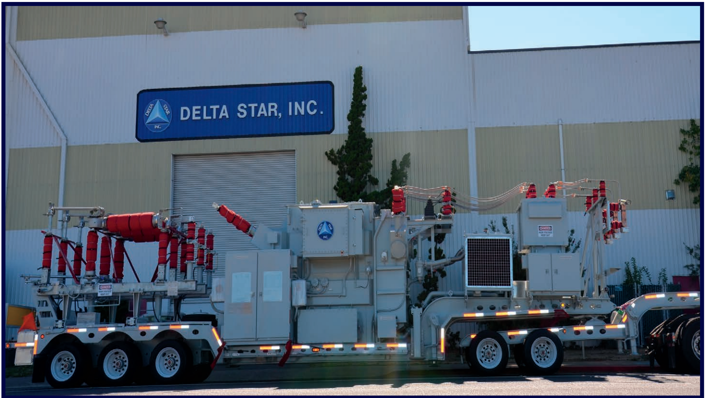
(10.5 MVA, 69 kV - 12.47 kV, LTC) 2016 | 56'-5" | 122,000 lbs. Customer Region: MIDWEST
