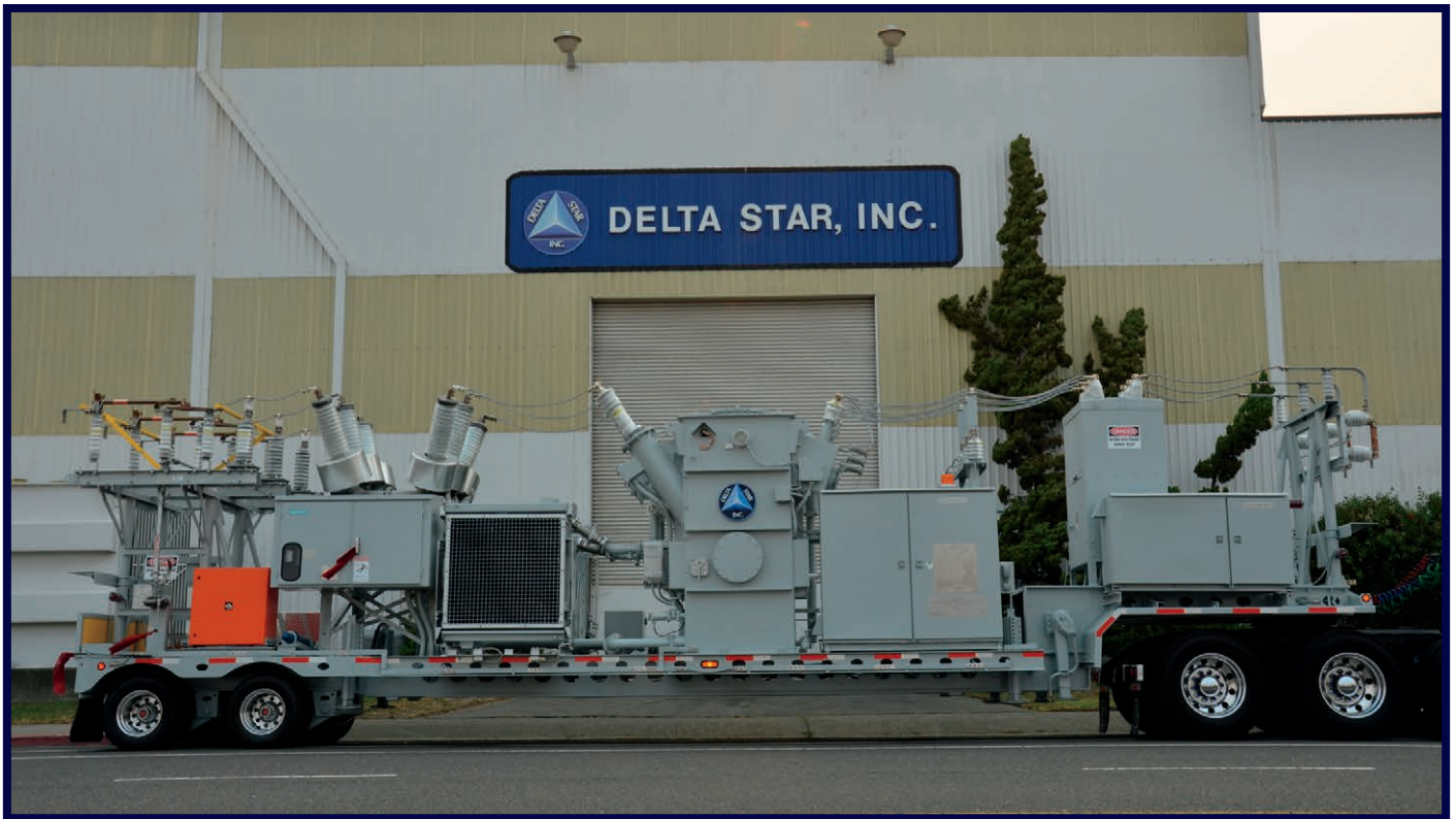
(14 MVA, 46 kV - 13.2 kV) 2017 | 44' | 83,000 lbs, Customer Region: MIDWEST
