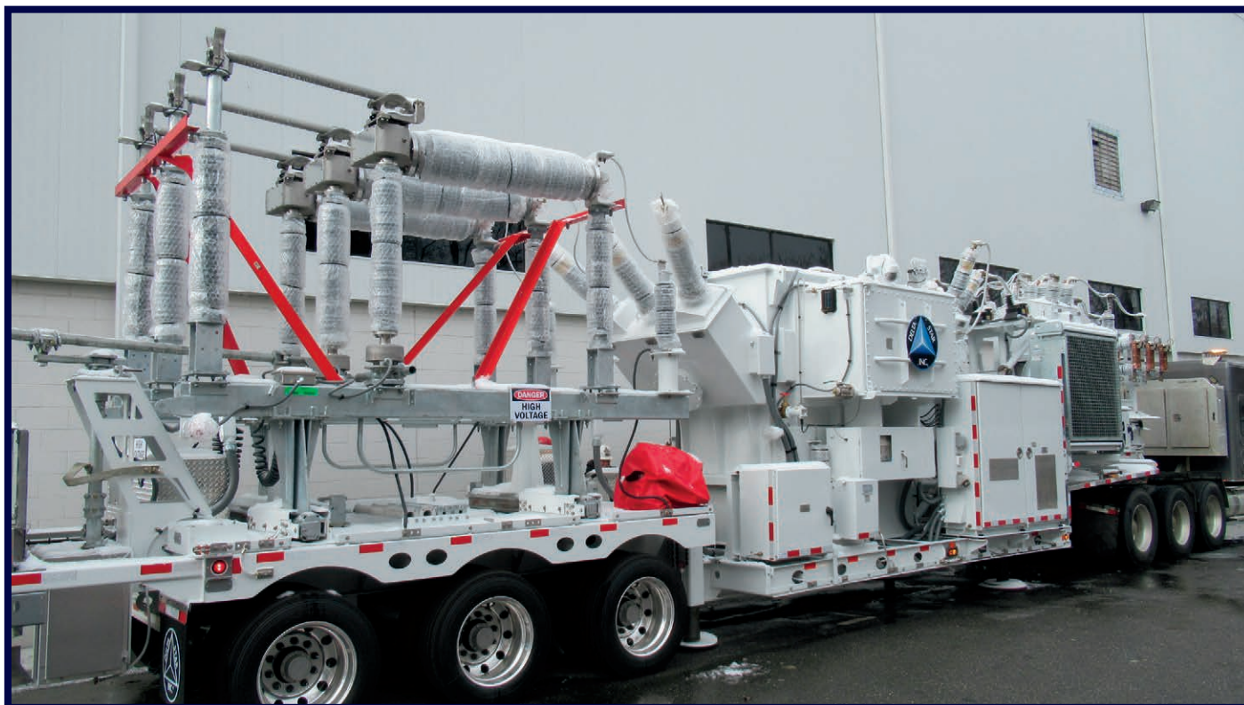
(20 MVA, 69 kV - 13.09 kV, LTC) 2018 | 48' | 112,000 lbs. LV Vacuum Breaker and HV Circuit Switcher Customer Region: MIDWEST
