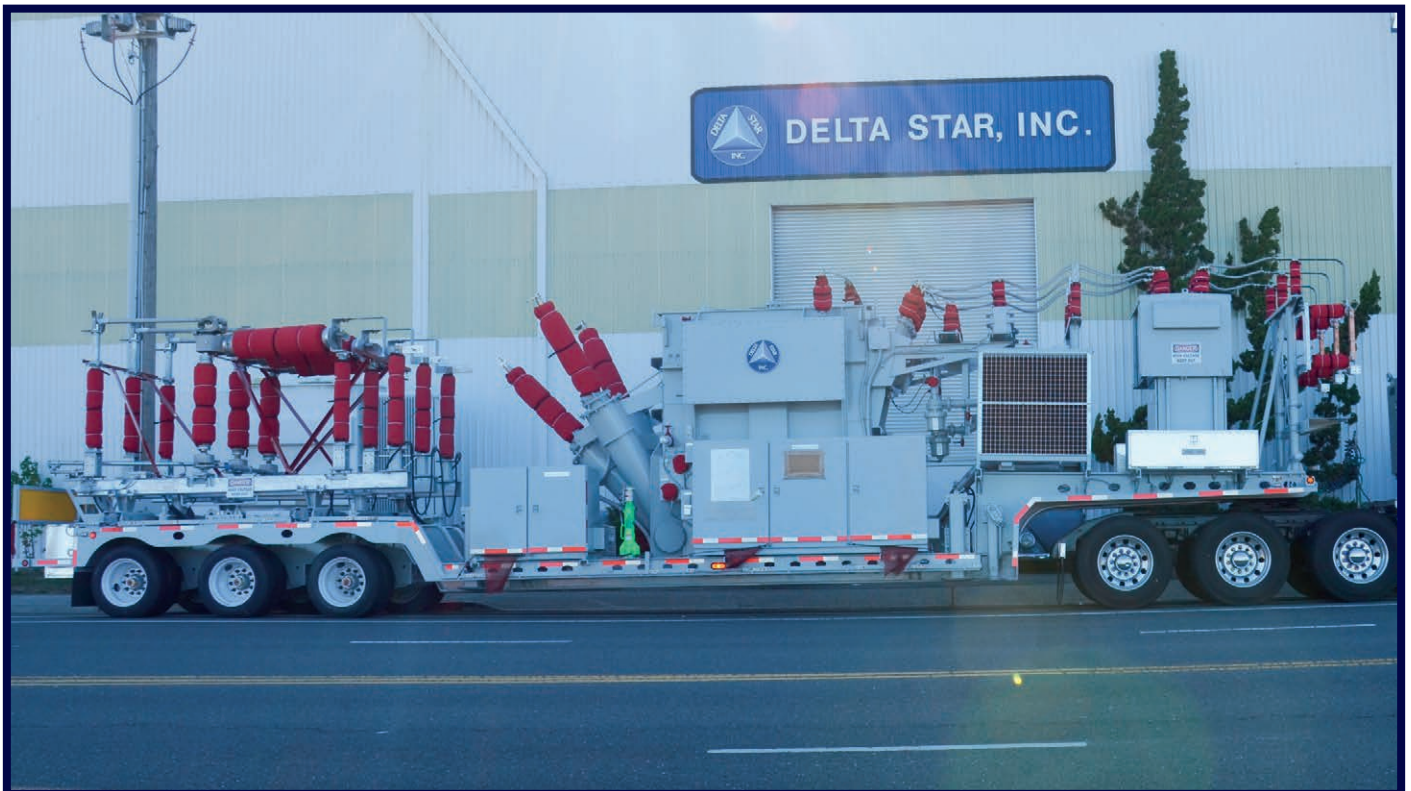
(20 MVA, 115.5 kV - 24.94 kV) 2015 | 50' | 118,000 lbs. Customer Region: WEST
