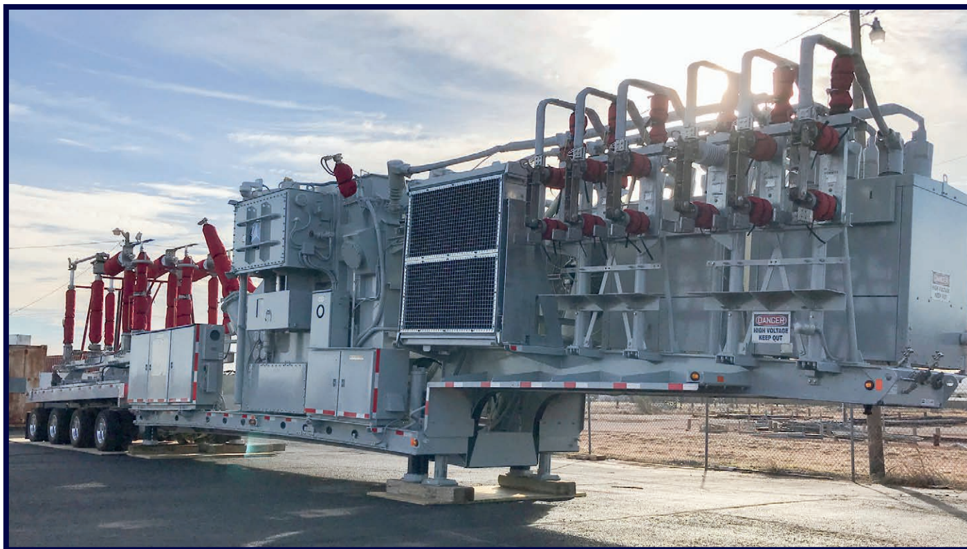
(35 MVA, 138 kV - 22.86 kV, LTC) 2018 | 65' | 180,000 lbs. Customer Region: WEST
