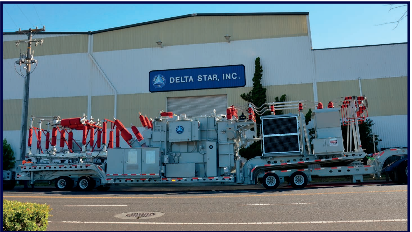
(30 MVA, 115 kV - 25 kV, LTC) 2017 | 78'-5" | 190,000 lbs. Customer Region: SOUTHEAST
