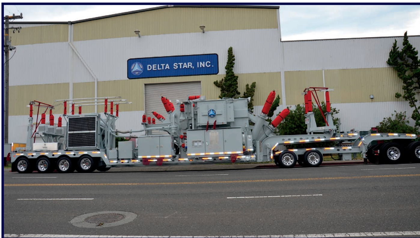
(40 MVA, 115 kV - 69 kV, LTC) 2017 | 65' | 134,000 lbs. Customer Region: MIDWEST
