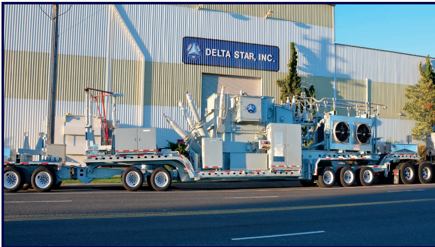
(50 MVA, 141 kV - 37.5 kV, LTC) 2015 | 59' | 176,000 lbs. Customer Region: WEST
