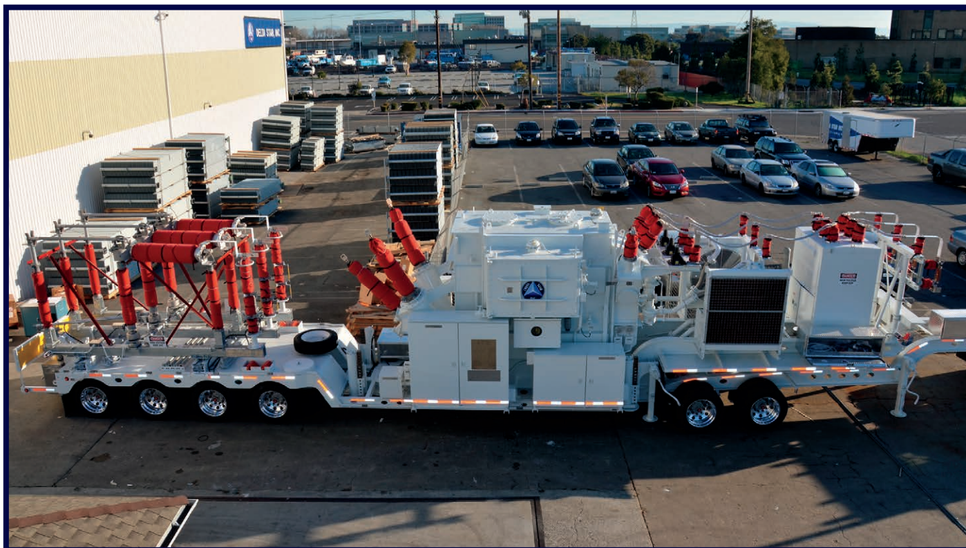
(30 MVA, 138 kV - 12.47 kV, LTC) 2014 | 64'-5" | 154,000 lbs. Customer Region: WEST
