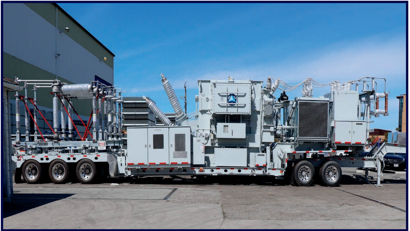
(25 MVA, 138 kV - 26.2 kV, LTC) 2018 | 64'-5" | 147,000 lbs. Customer Region: MIDWEST
