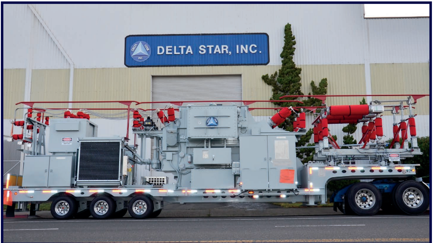
(20 MVA, 67 kV - 26.4 kV, LTC) 2017 | 46' | 120,000 lbs. Customer Region: WEST
