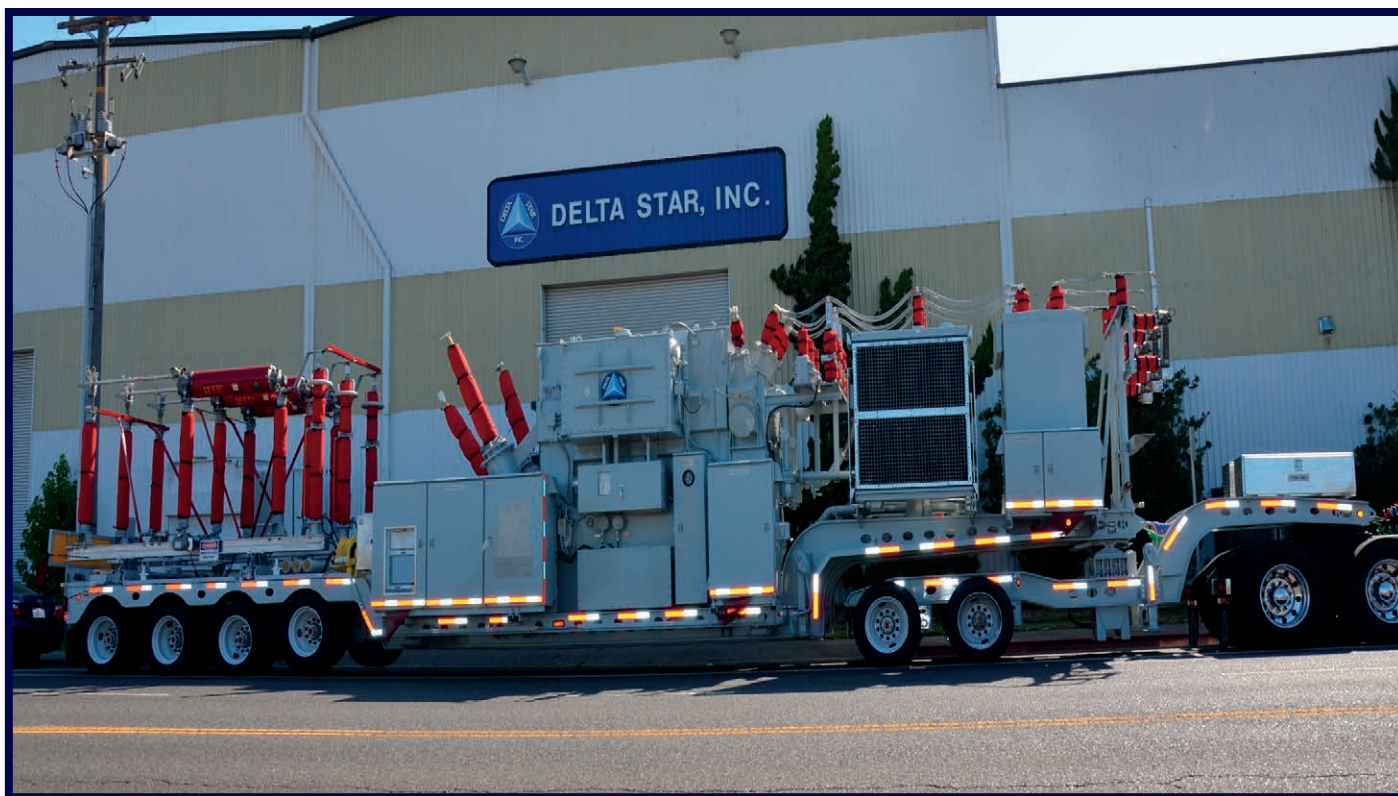
(25 MVA, 69 kV - 26.4 kV, LTC) 2017 | 66'-5" | 162,000 lbs. Customer Region: MIDWEST
