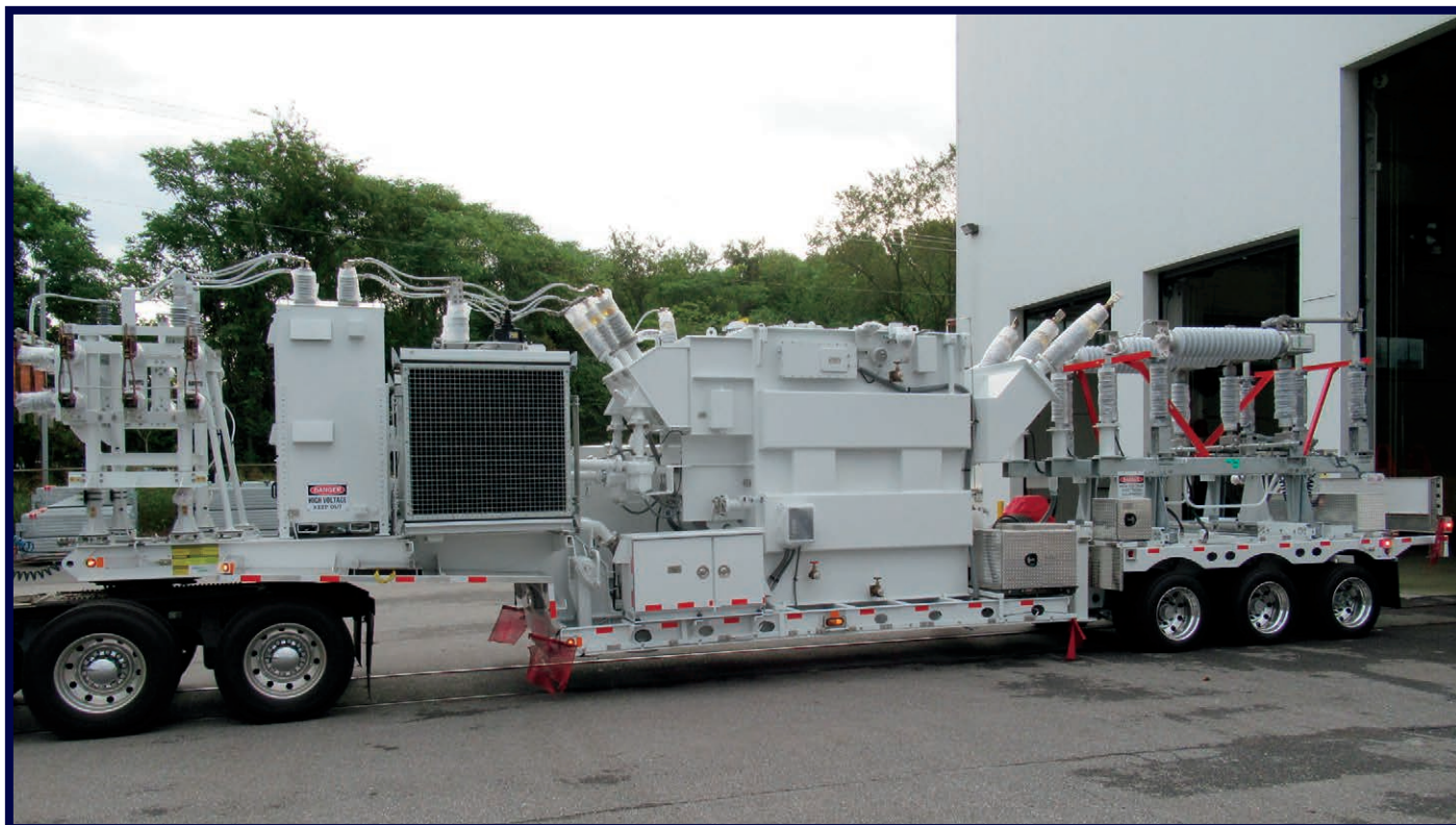
(20 MVA, 69 kV - 13.09 kV, LTC) 2018 | 46' | 112,000 lbs. LV Vacuum Breaker and HV Circuit Switcher Customer Region: WEST
