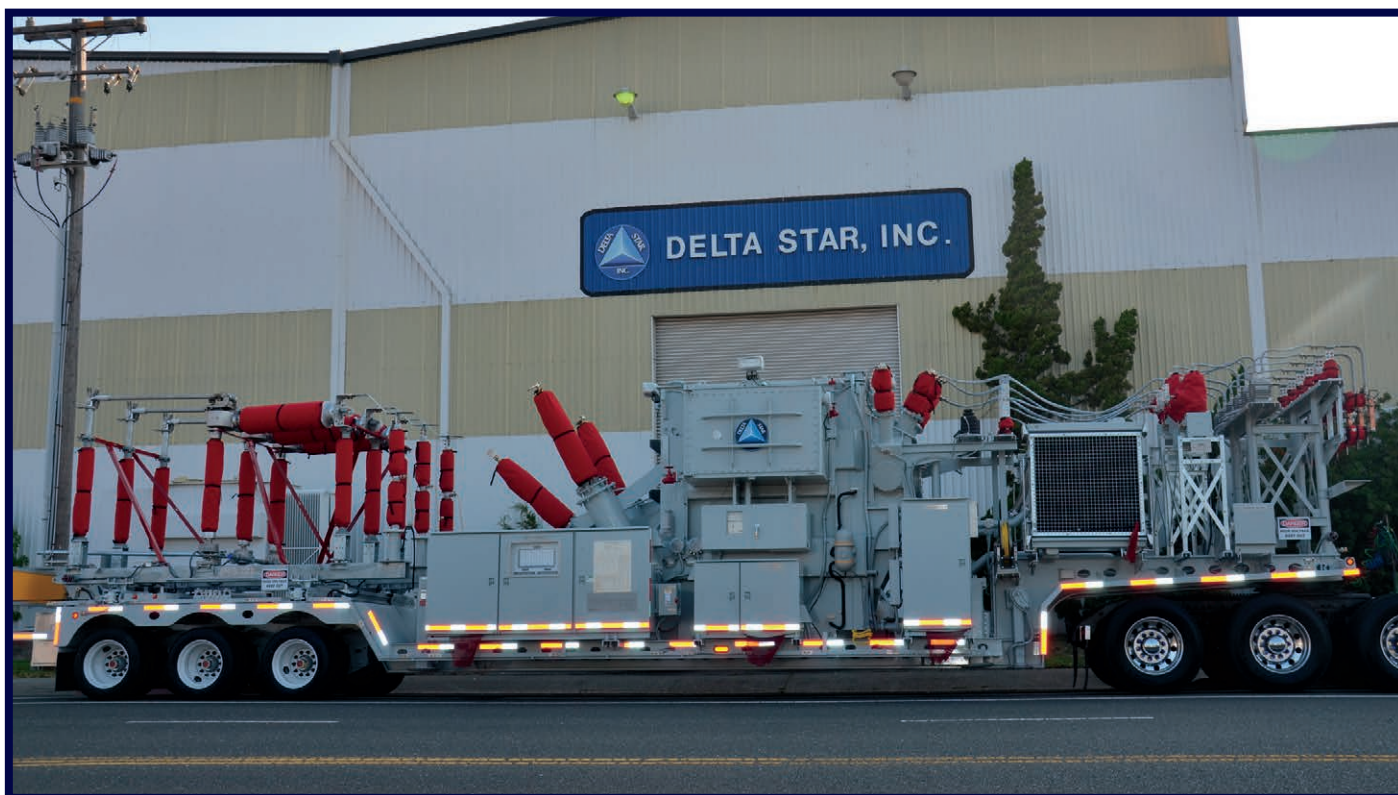
(15 MVA, 134 kV - 12.47 kV, LTC) 2017 | 62' | 119,000 lbs. Customer Region: MIDWEST
