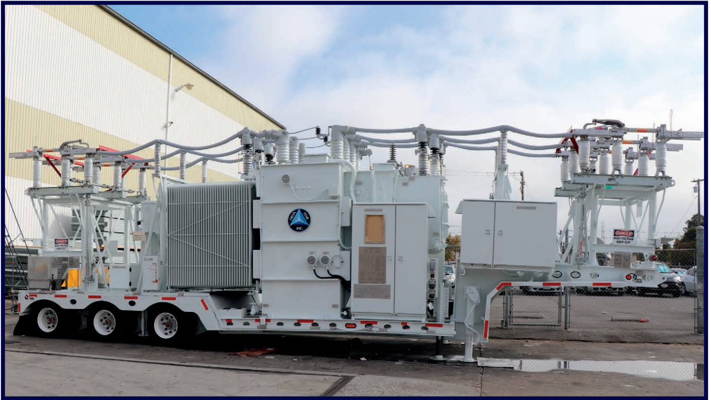
(4 MVA, 34.5 kV - 34.5 kV, LTC) 2018 | 40' | 125,820 lbs. Customer Region: MIDWEST
