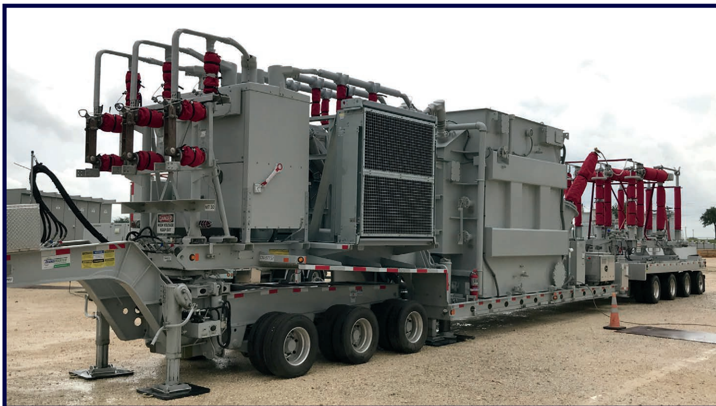
(50 MVA, 138 kV - 26.4 kV, LTC) 2018 | 72' | 179,000 lbs. Customer Region: WEST
