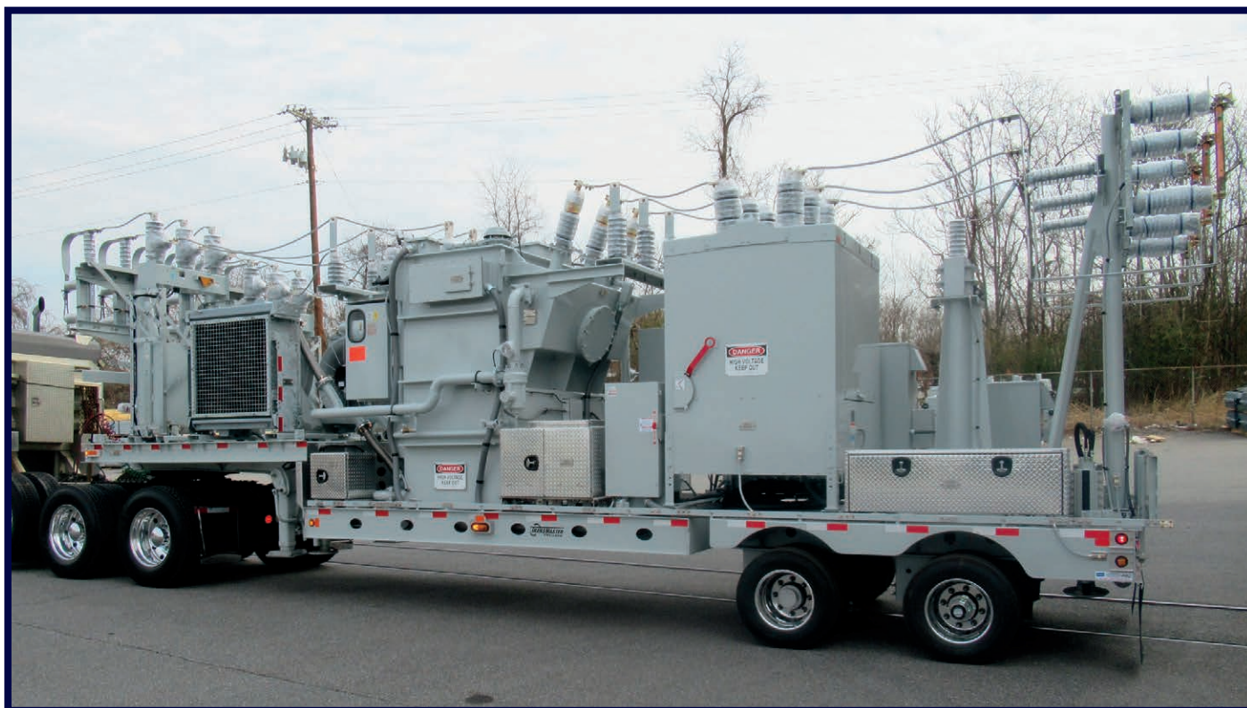
(6 MVA, 34.5 kV - 13.2 kV, LTC) 2018 | 33' | 77,000 lbs. LV Vacuum Breaker and HV Recloser Customer Region: MIDWEST
