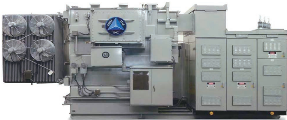
UNITIZED SUBSTATION (SKID MOUNTED)
