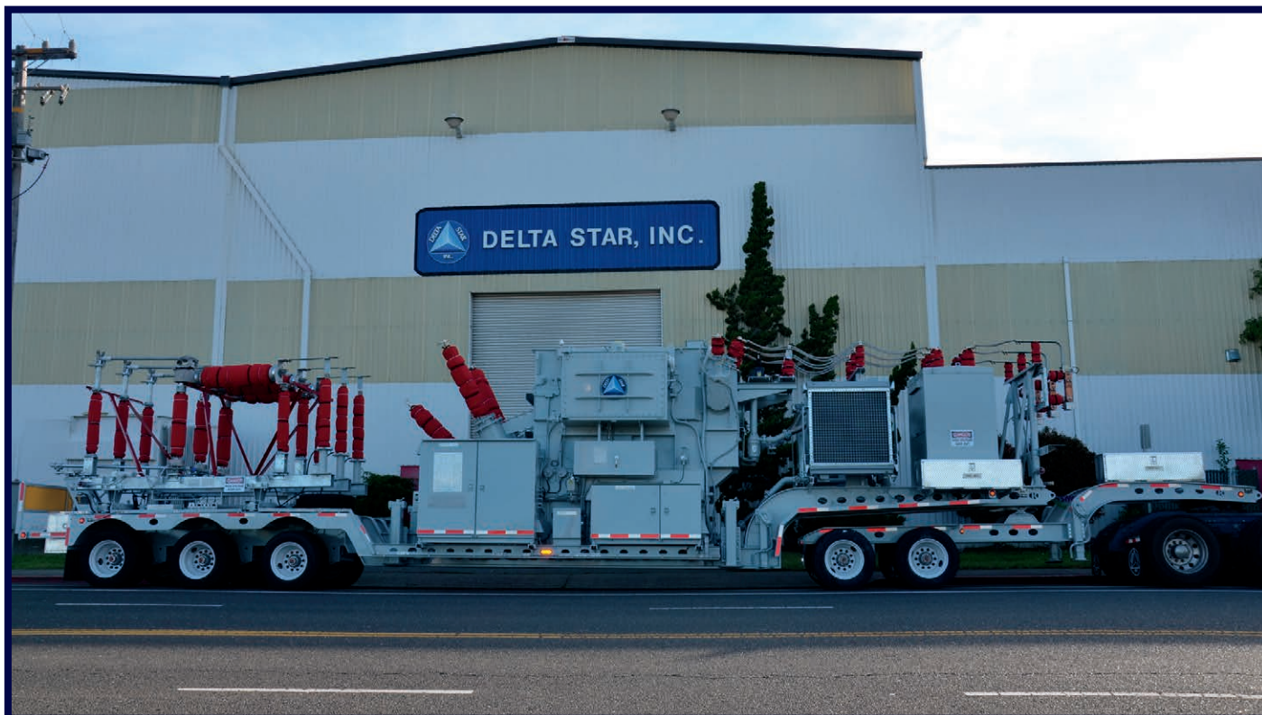
(25 MVA, 115 kV - 12.47 kV, LTC) 2016 | 52' | 142,000 lbs. Customer Region: WEST
