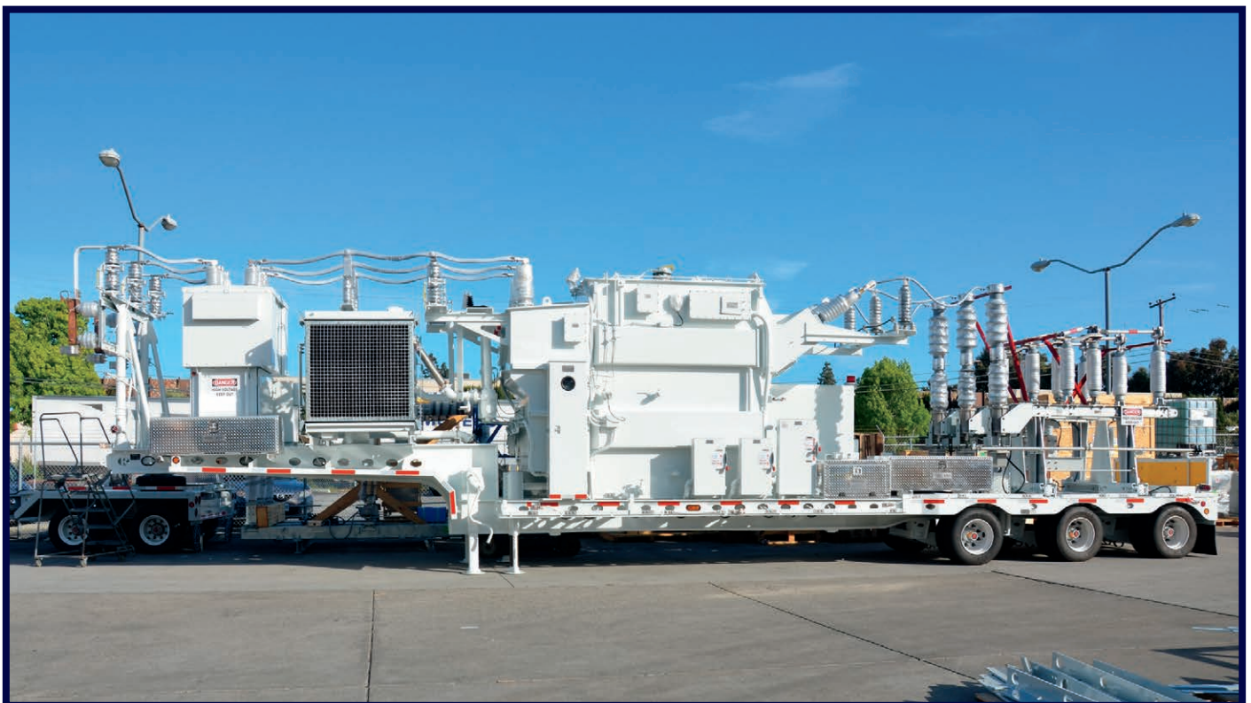
(14 MVA, 45 kV - 13.09 kV, LTC) 2017 | 54' | 123,400 lbs. Customer Region: SOUTHEAST
