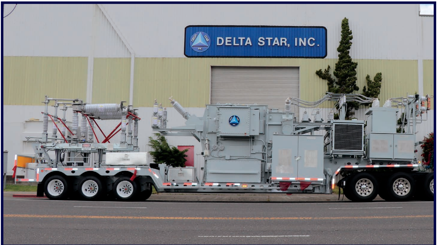
(10 MVA, 69 kV - 1,309 kV, LTC) 2018 | 48' | 112,000 lbs. Customer Region: MIDWEST
