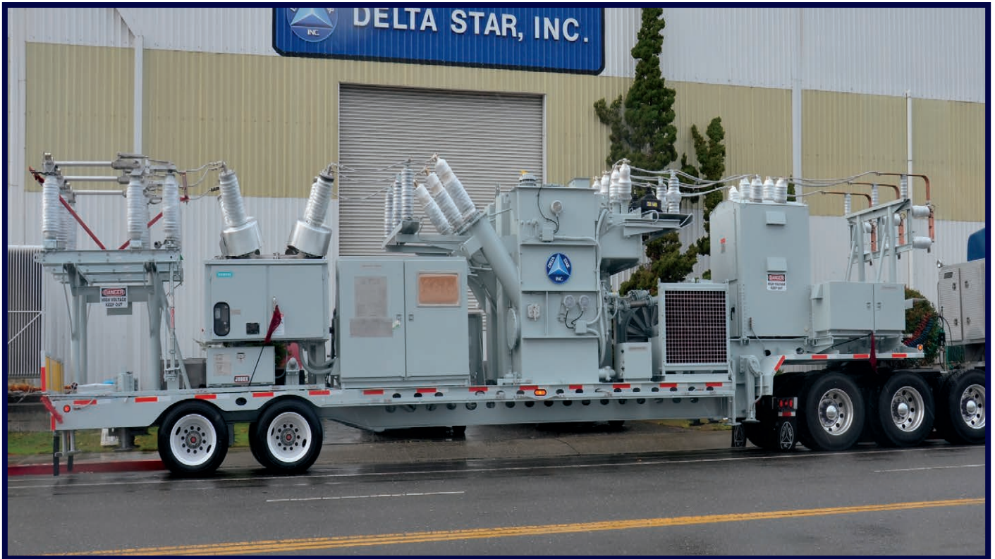
(15 MVA, 69 kV - 24.94 kV) 2015 | 44' | 91,000 lbs. Customer Region: MIDWEST
