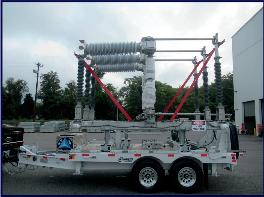
Mobile Circuit Switcher Trailer Customer Region: SOUTHWEST
